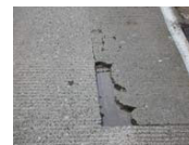
Pothole on I-5
