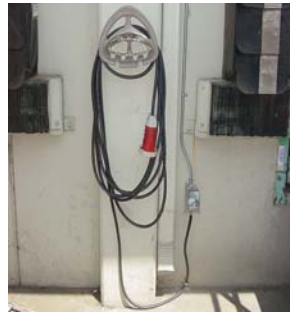
Shore Power: 208 Volt, Single Phase
