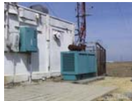
Remote communications center generator
