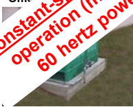
Hospital emergency generator
